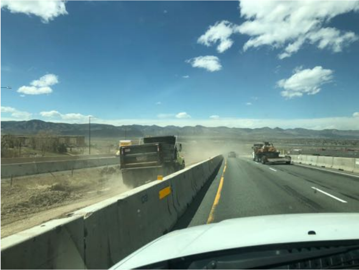
Figure 12: Dust resuspended by construction on C-470 on a breezy day April 12 th . Note the dust kicked up by the dump truck's tires, and a bulldozer ahead raising enough dust to create a visibility hazard.
